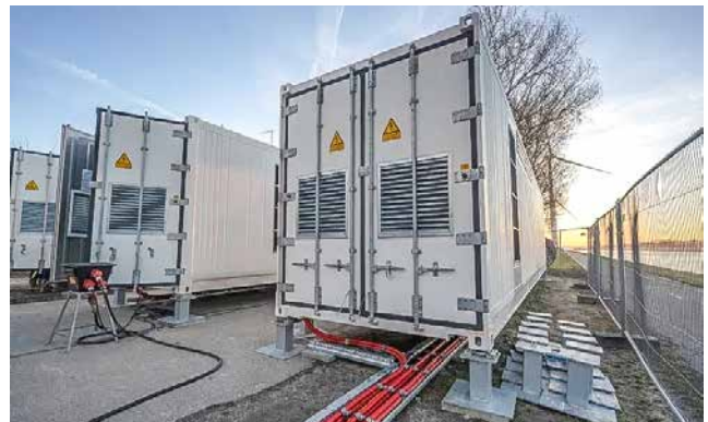
Industrial battery installation
